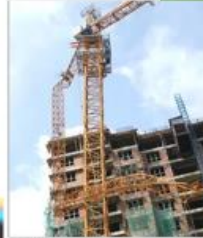
Collapsed tower crane
