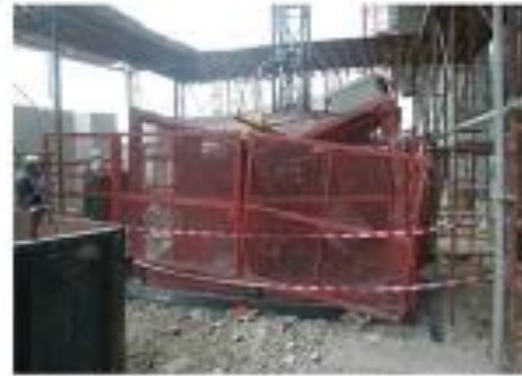
Collapsed passenger lift
